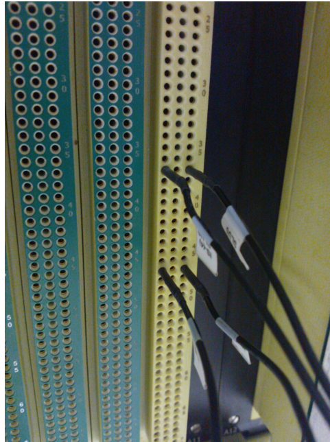
Figure 3-5 I Sense Pins of CEDGN Load Card Cable U8972-61628 are manually probed to ICA Slot 10
